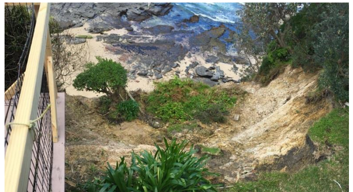
Berrara landslide caused by the August 2015 storm
