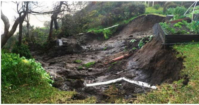
Mollismook landslide caused by the August 2015 storm
