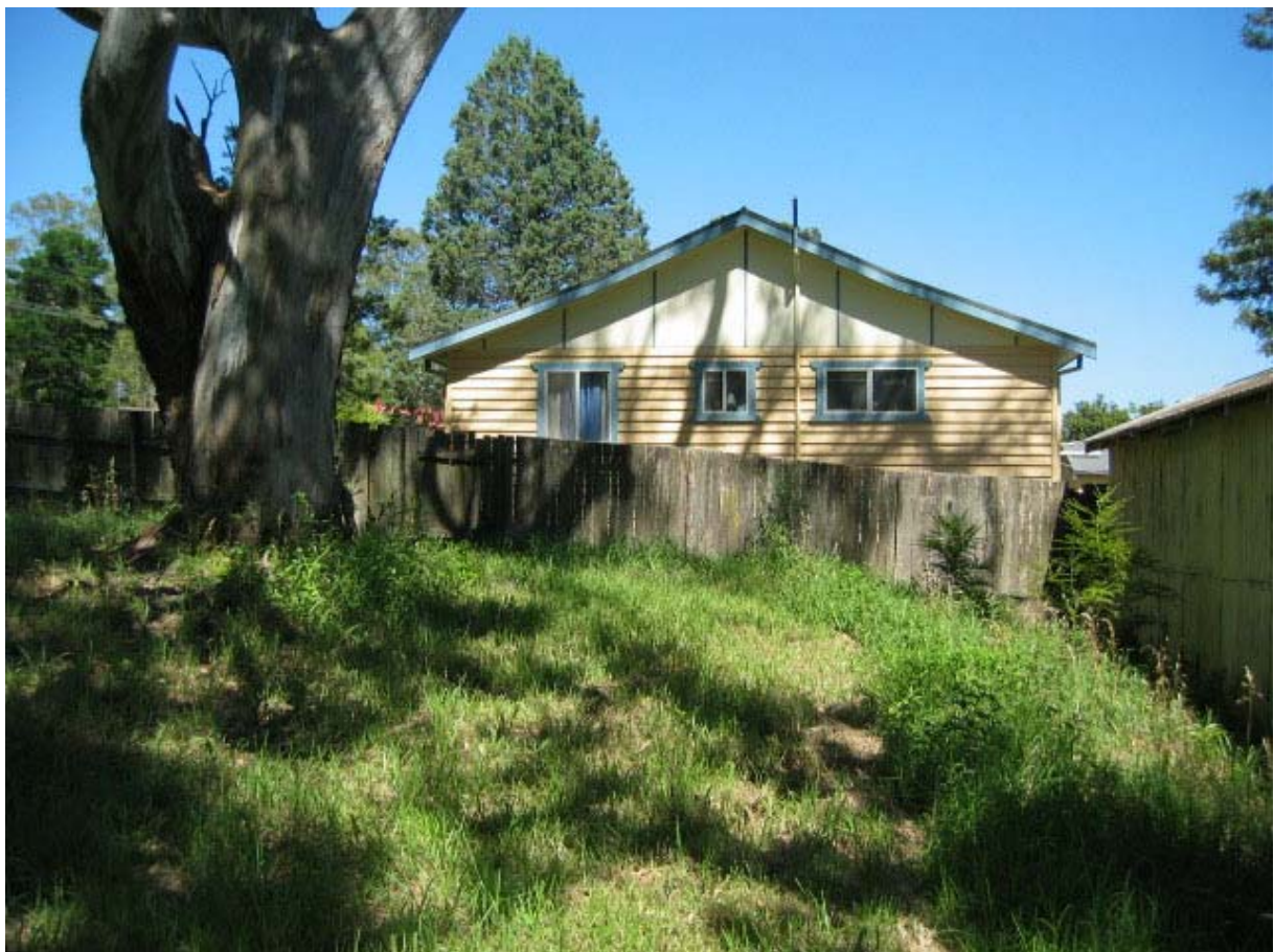
Figure No.B11: Garage and sheds to the rear of the Caretaker's Cottage. Figure No.B12: East elevation of the Caretaker's Cottage.
