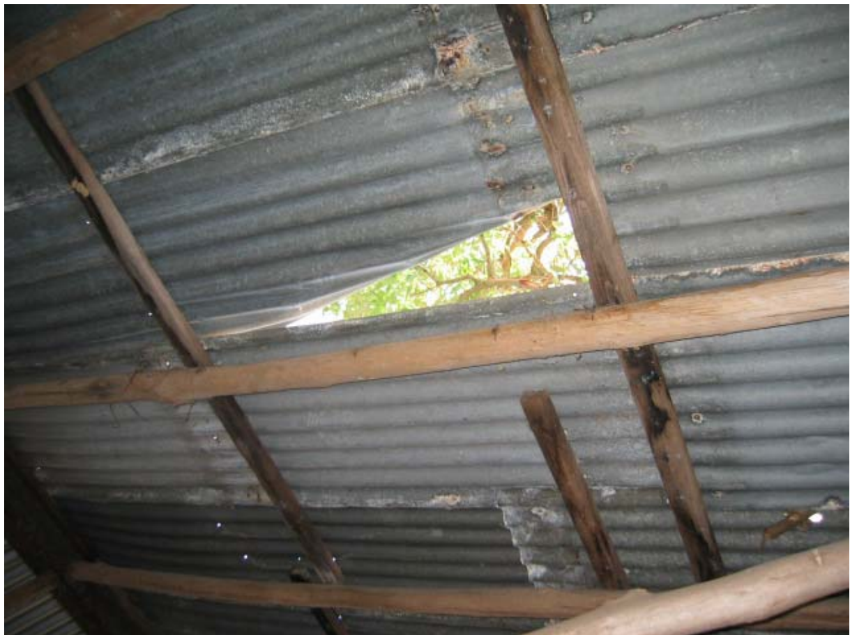
Figure No.B60: Poultry Pavilion, interior. Figure No.B61: Damage to roof of Poultry Pavilion.
