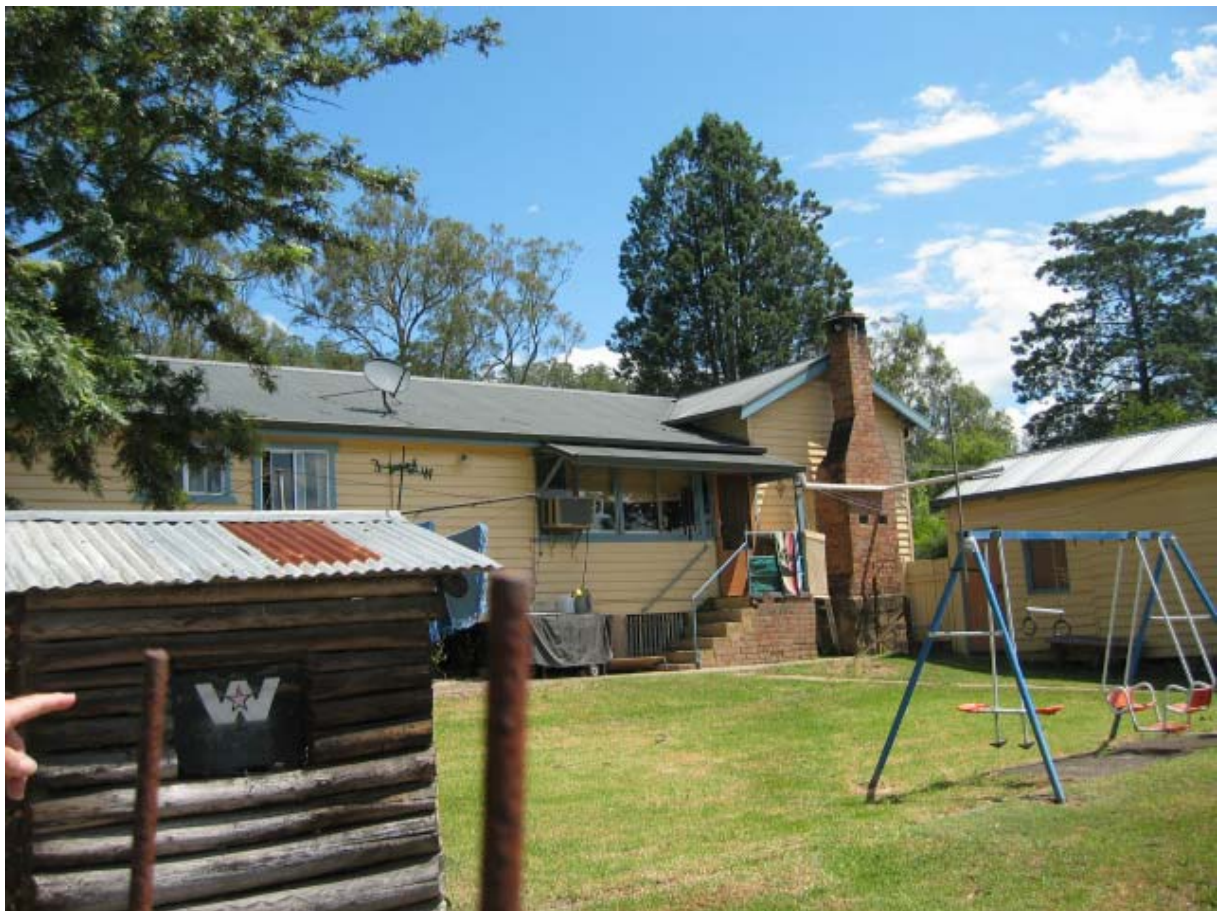
Figure No.B9: Front (south) elevation of the Caretaker's Cottage. Figure No.B10: Rear (north) elevation of the Caretaker's Cottage.
