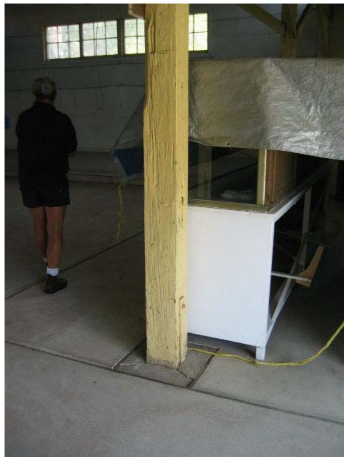
Figure No.B30: General view of interior of Agricultural Pavilion. Figure No.B31: Detail of post.
