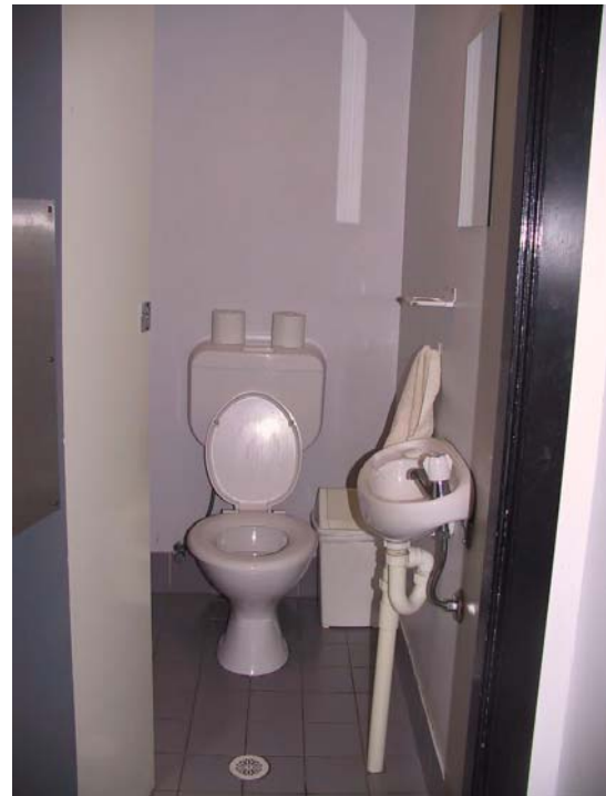
Figure No.23: Toilet.
