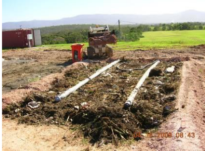
HDPE pipes for the Forced Aeration Compost System
