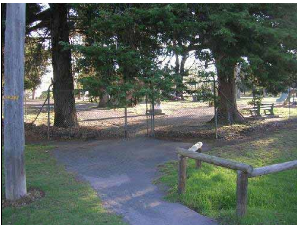
Figure 9. The main pedestrian entry way for people coming from the business district presents poorly.
