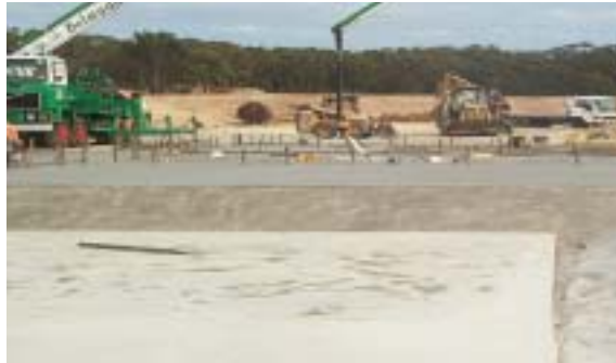
Culburra – Storm Pond Sump
