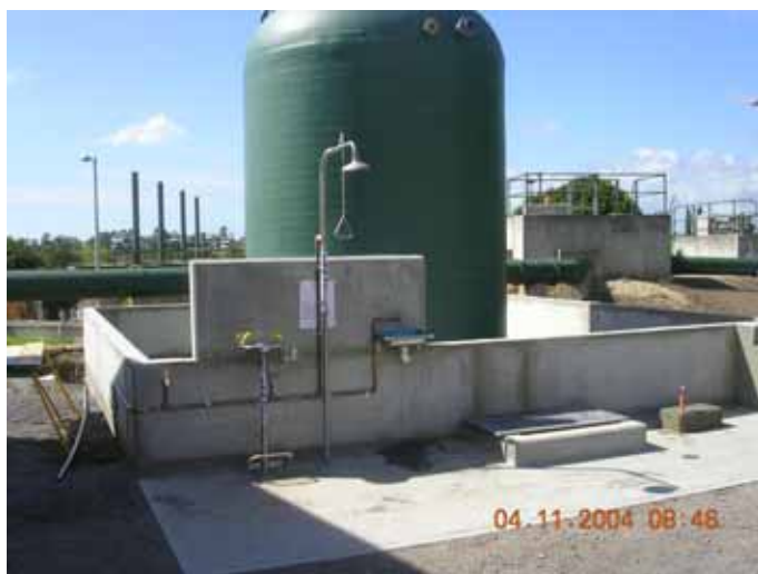
Ferric chloride tank, bund and safety wash at Bomaderry STP
