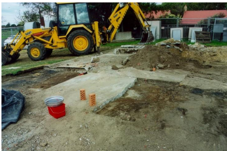
Figure 21: (middle) The lowest layer of concrete. The original ground surface can be seen to the left and right of the slab of concrete remaining in place.
