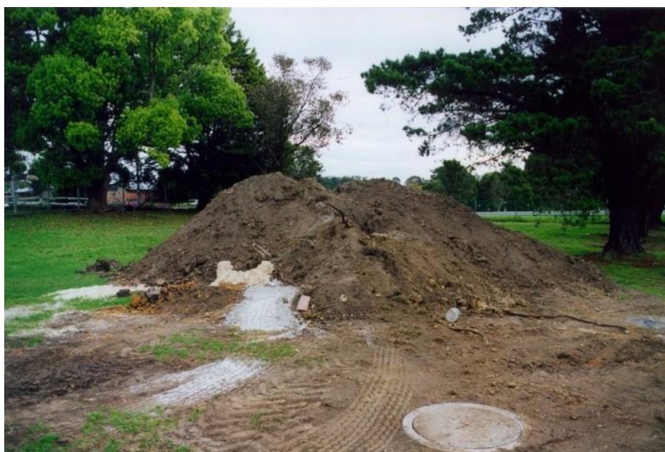
Figure 3: Soil from footings for additions to the Tourist Information Centre to provide disabled person's access (8 th September 1999).
