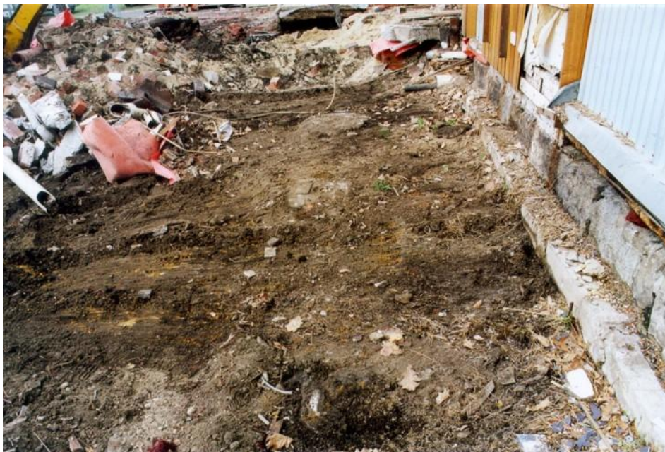
Figure 25: The footings of the foundations of the old Prague Lodge were left in place during the demolition. It is considered that the original ground layer associated with Graham Lodge is present. Relics are present in this area.
