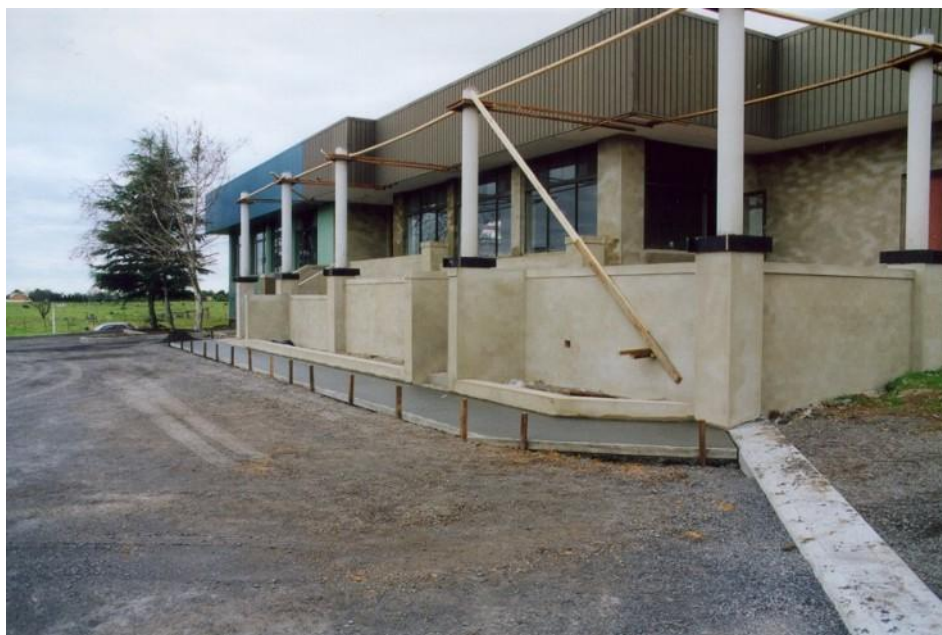
Figure 2: Additions to the Tourist Information Centre to provide disabled person's access (8 th September 1999).
