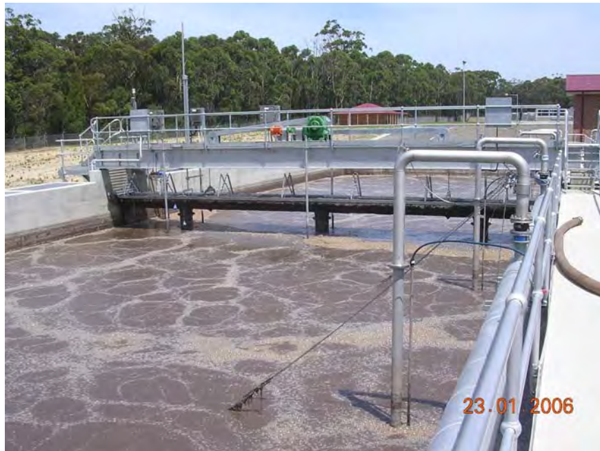
Ulladulla STP Aeration Tank
