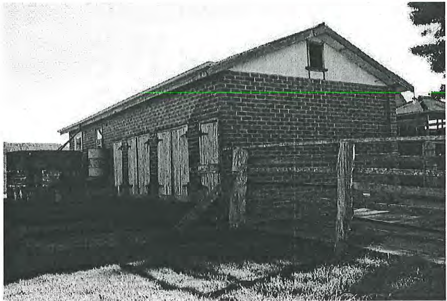
1950's bails, 2x2, 2x1, exit onto concrete, louvred gable for ventilation to roof area. Water tank for dairy use. Looking north-west. MH 1997 photograph 2 6
