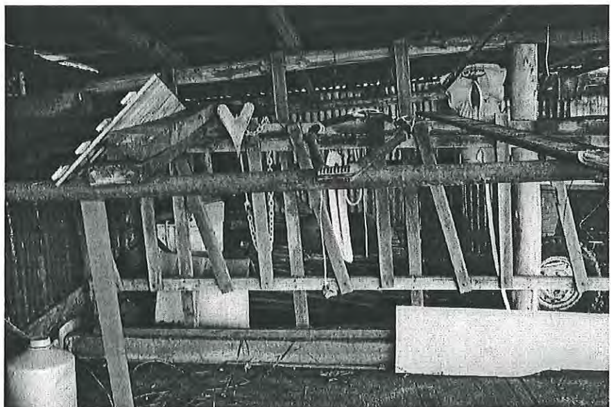
Feed stalls adjacent to chaff cutting area. Five bails, no boxes remain. Looking west MH 1997 photograph 9.22
