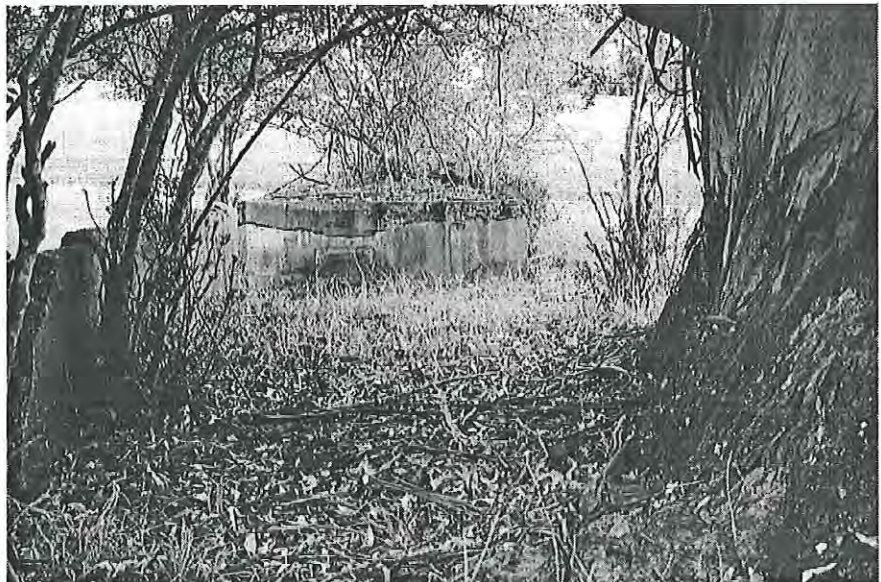
Concrete plinth showing recess for floor joists, concrete wall. Looking east MH 1997 photograph 7.21
