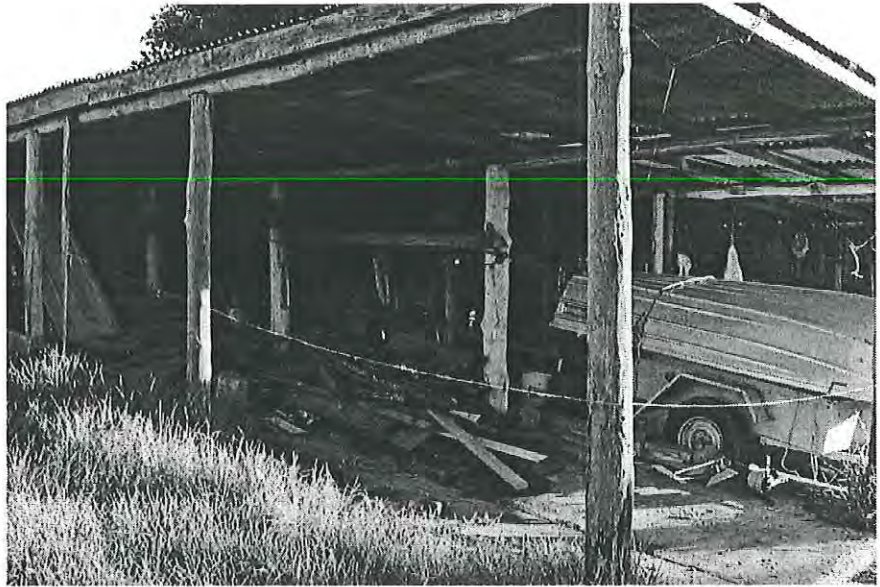
Feed stalls, sawn timber frame and corrugated iron roof, supported on natural round posts 6-8 inches diameter, concrete floor. Looking south-west MH 1997 photograph 9.23
