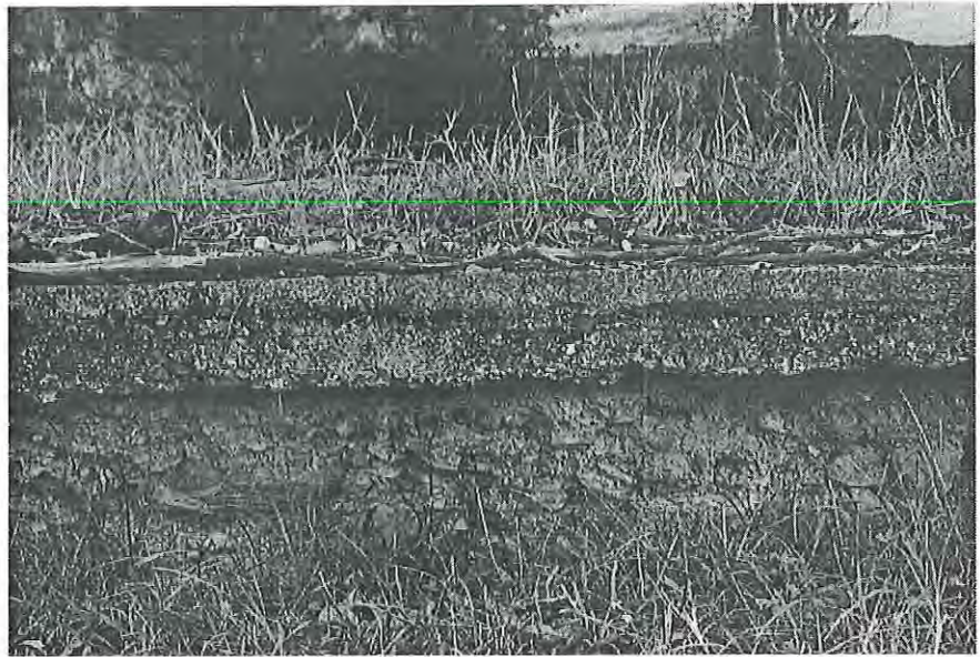
Detail of concrete factory floor on earth terrace. Looking north MH 1997 photograph 7.23
