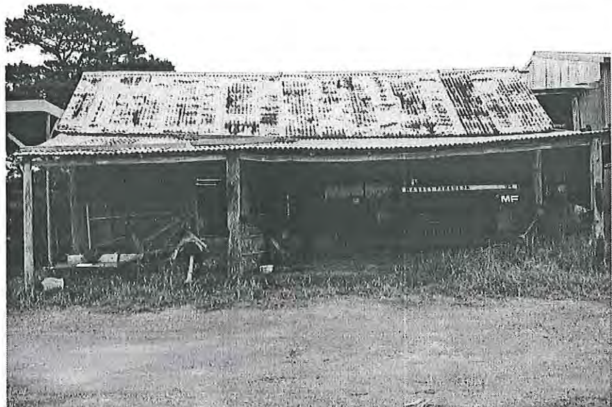
Timber slab, corn shed, indicating fodder cropping. Rebuilt, originally had loft. Looking west MH 1997 photograph 4.2
