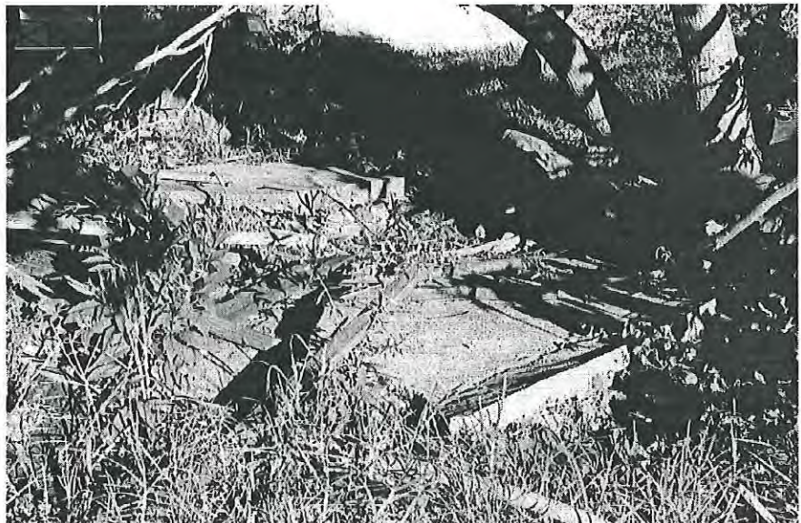
Concrete foundation for chaff cutting and fodder storage. Looking south-east MH 1997 photograph 9.21
