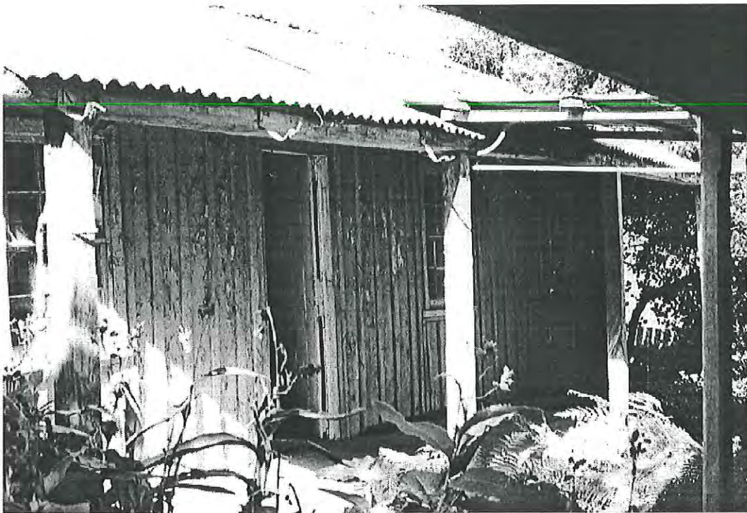
Above: Western elevation. Vertical sawn plank and batten house with timber 6 pane double sash windows, encircling timber verandah. Looking east MH 1997 photograph 7.5
