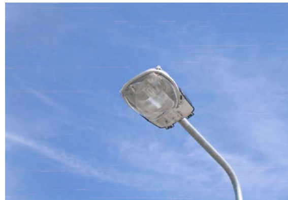
CFL luminaire after installation
