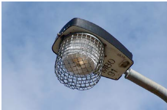
An old 80W MV luminaire
