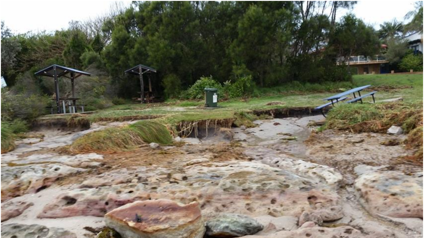
Currarong Rock Pools; sand loss and park asset damage
