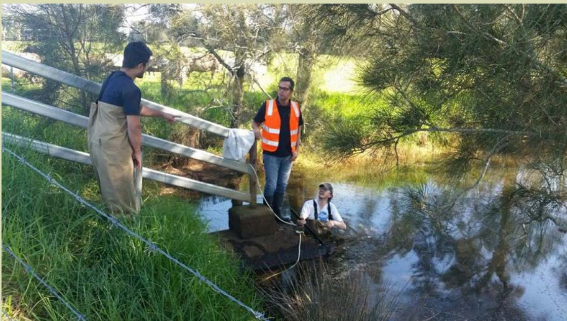
WRL staff installing flow monitors for new tidal gate and assessing maintenance requirement
