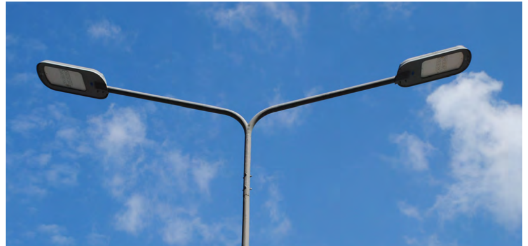
LED Street Lights
