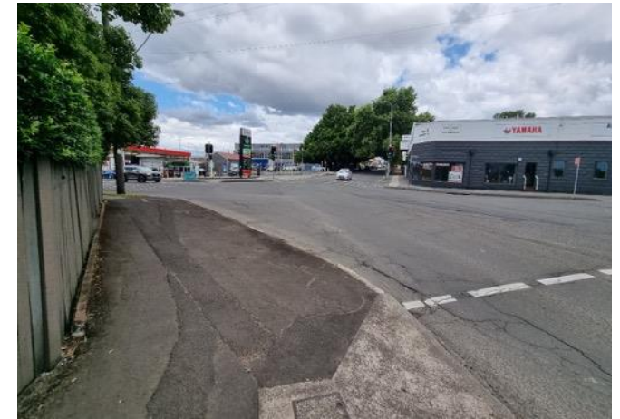
Figure 38: Uneven pedestrian surface along Bridge road (Source: CrossleyTP, 2022)
