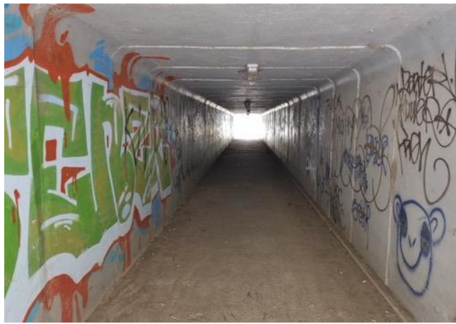
Figure 40: Unattractive environment at underpass of Campbell Place (Source: CrossleyTP, 2022)
