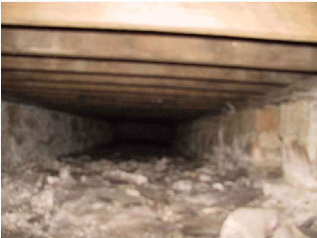
Figure No.44 & 45: The sub-floor area below the supper room
