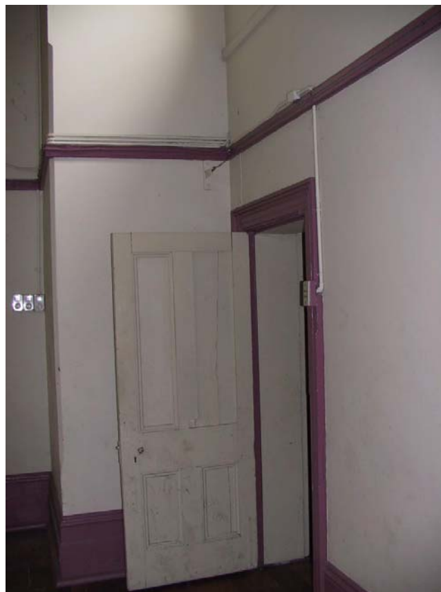
Figure No.37: The western wall of the Lodge room showing the door to the rear addition which is no longer in use.
