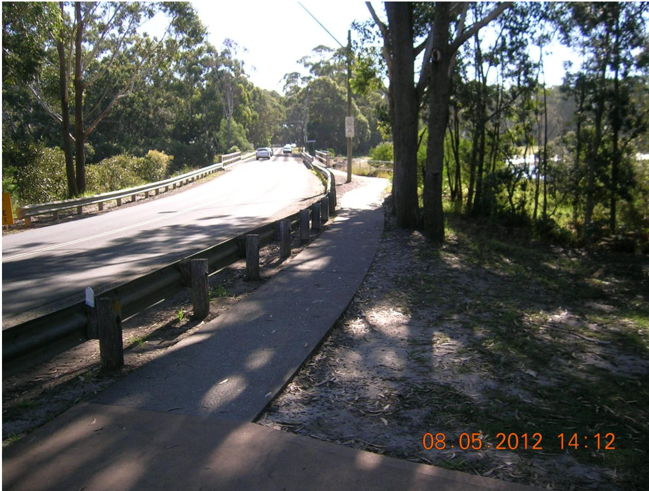
Figure 15 - Narrow Moona Moona Creek pedestrian bridge which requires further assessment
