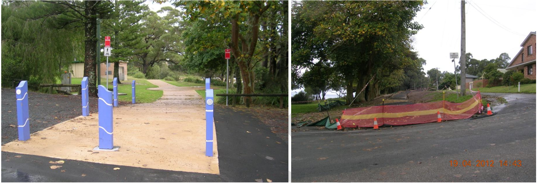
Figure 18 - Holden Street boat ramp pedestrian crossing which requires further assessment
