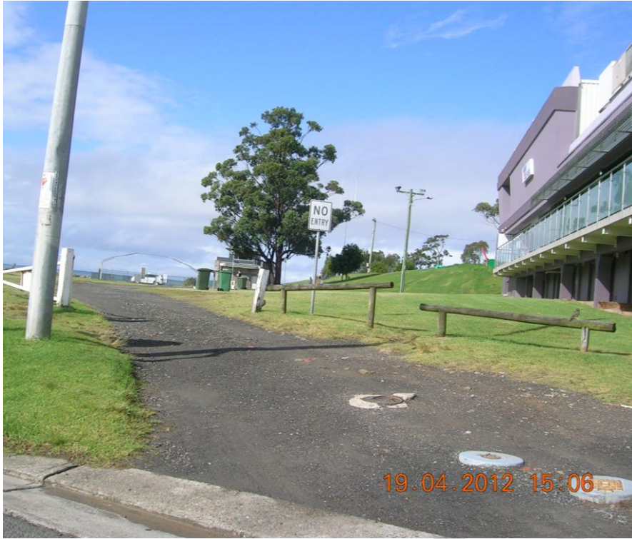
Figure 12 - Missing section of shared path between Huskisson Wharf and Voyager Park amenities building
