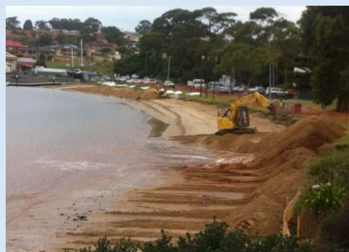
Ulladulla Harbour – beach scraping post June 2016 storm
