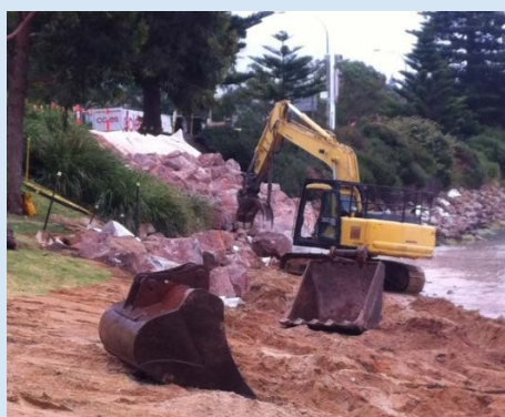
Ulladulla Harbour – repair rock protection post June 2016 storm
