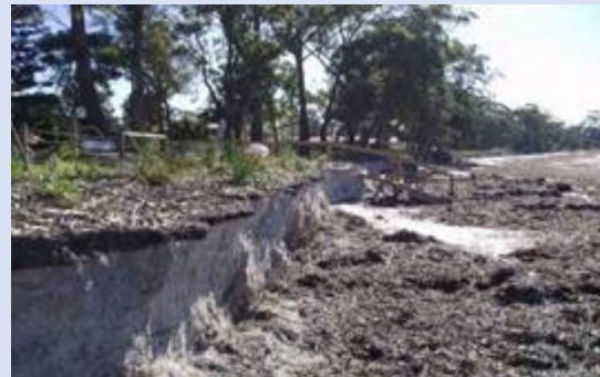
Callala Bay - erosion post storm 2005
