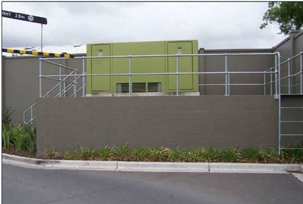
Figure 51 - Example substation raised above 1:100 flood level
