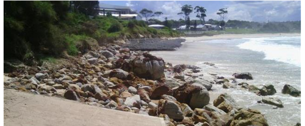
Late 2015 showing major erosion and exposure of gabion revetment toe
