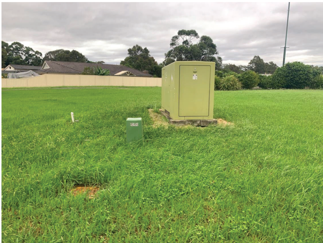
Photograph 11: Electrical substation at corner of Burradoo Crescent and Kardella Avenue looking west.
