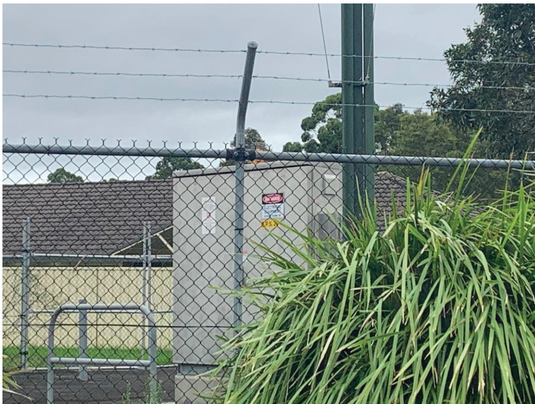
Photograph 13: Close up of electrical storage facility at north-west corner of site.
