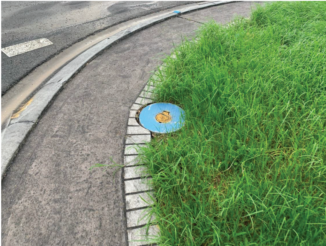
Photograph 5: Services at Carrington Park Drive and Old Southern Road intersection at the southern portion of site.
