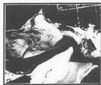
F = flood scoured
