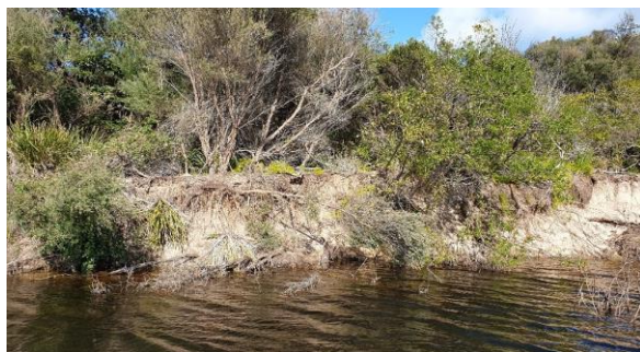
Ongoing erosion along inside of bend, Swan Lake inlet channel
