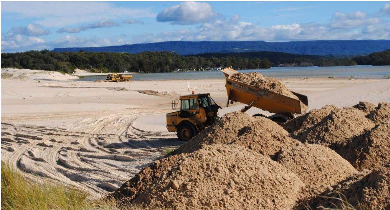
Figure 5-14: Contractors placing sand near northern dunes after removing it from the entrance of Lake Conjola on 13 June 2019 (source: Illawarra Mercury)
