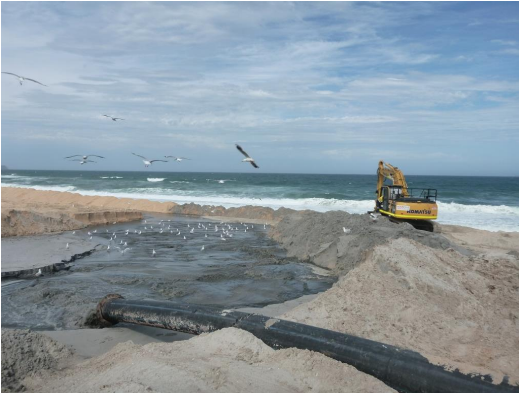
Figure 5-21: Management of sand slurry discharge within a bunded beach area at Blacksmiths Beach
