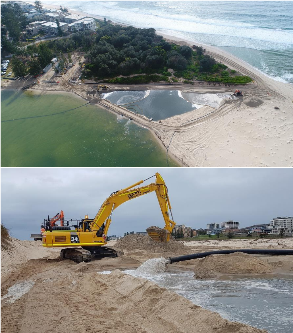
Figure 5-20: Management of sand slurry discharge within a bunded beach area at The Entrance, Central Coast
