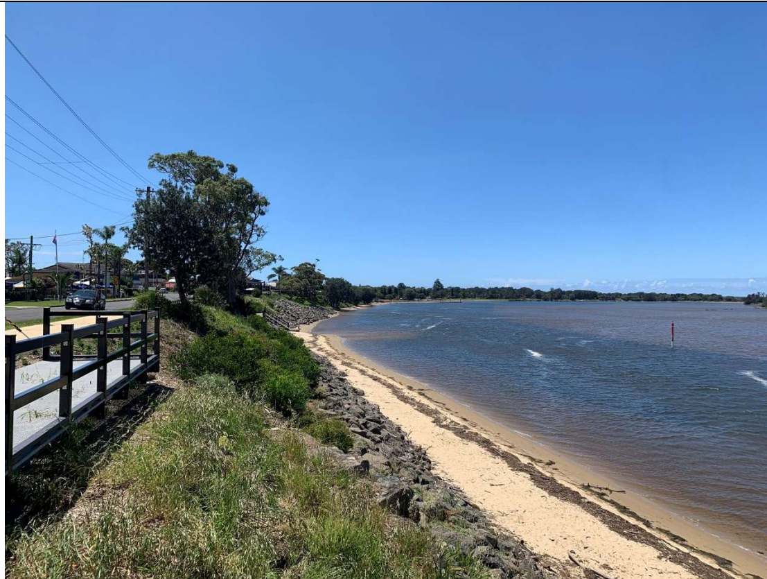
Plate 8: Middle portion of River Road Reserve. A rock revetment wall occurs along this section of the reserve.
