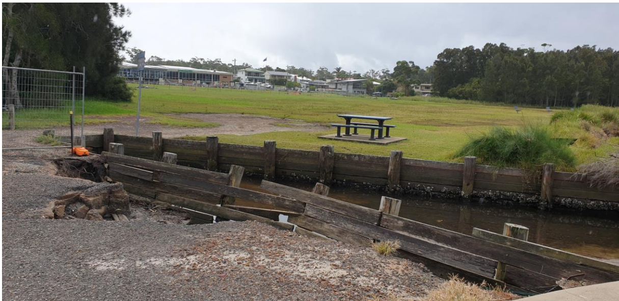
Figure 4-42 – Lions Park foreshore with erosion damage to timber retaining wall at boat ramp fishing table (16 March 2022). Site reference S013.
