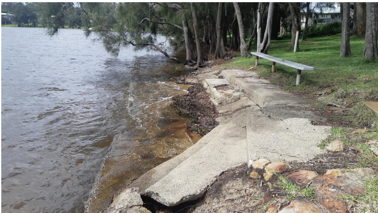
Figure 3-19 – Seating and concrete foreshore access area being undermined by erosion (Blackett Reserve, 28 November 2021). Site reference STB01.
