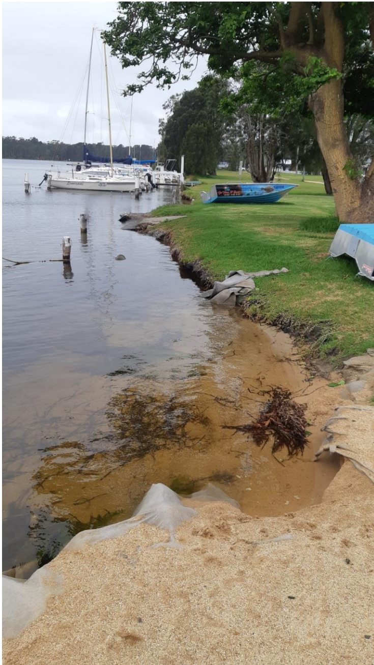
Figure 4-29 – Typical foreshore area upstream of Nielson Lane boat ramp, looking east. Note private mooring and vessel launching structures and failed geotextile bank protection (27 November 2021). Site reference S004.
