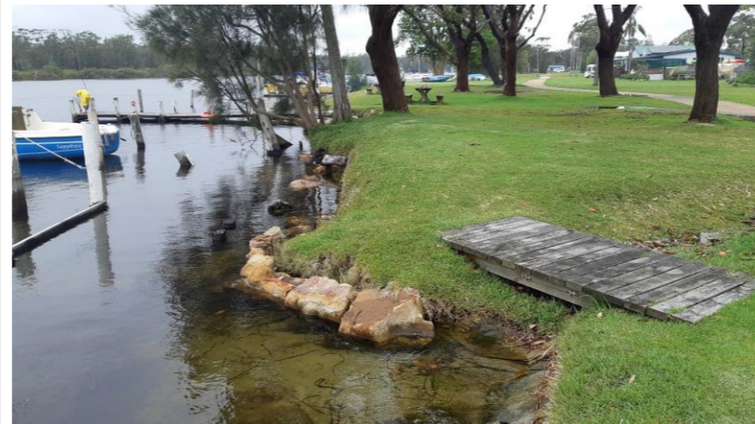
Rocky foreshore with some undermined casuarinas Site Ref S004
