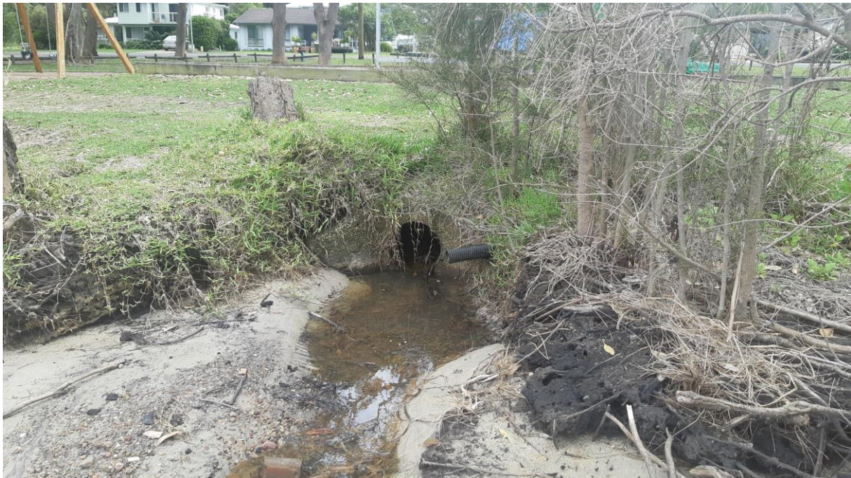
Figure 6-10 – Stormwater outflow at Berrara Lagoon reserve contributing to foreshore erosion (1 December 2021). Site reference BC05.
