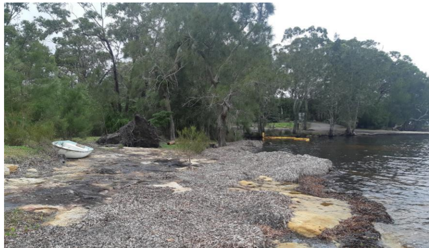
Undermined tree at Wrights Beach Site Ref WB01
