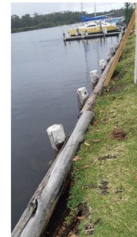
Sinkholes forming behind timber seawall Site Ref S004
