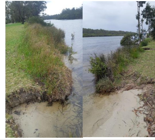
Eroded foreshore at Jacob Elimoos Reserve
