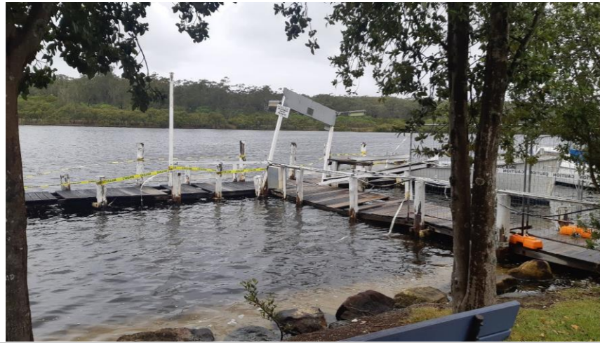
Damaged mooring structures near Sussex Inlet RSL
