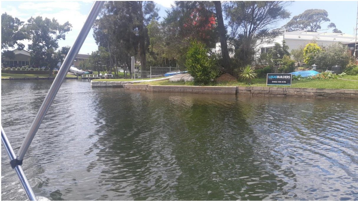
Figure 4-43 – Damaged retaining wall at Sussex Inlet Quays (7 December 2021) Site reference S010.
