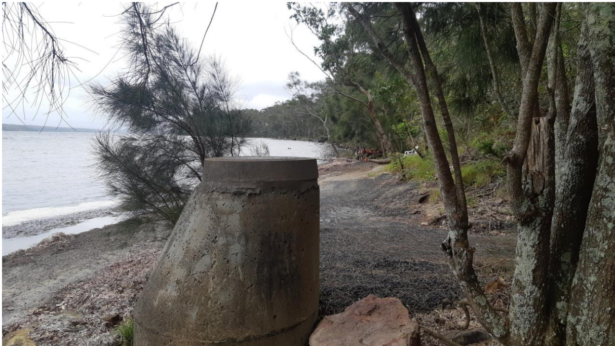
Figure 3-26 – Macleans Point foreshore looking west (28 November 2021). Top – area of active bank erosion where established riparian vegetation has been undermined. Bottom – sewer infrastructure and Basin walking track within area subject to inundation. Site reference MP01.
