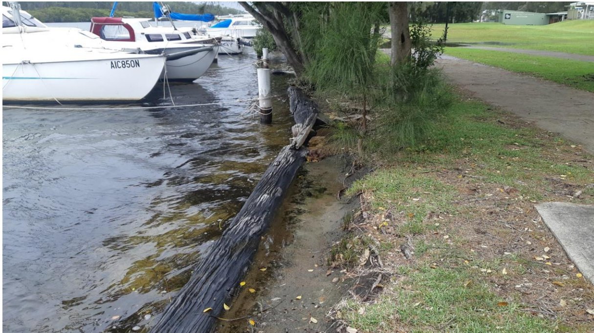
Figure 4-39 – Foreshore near Sussex Inlet RSL club showing erosion behind timber log bank protection (27 November 2021). Site reference S007.
