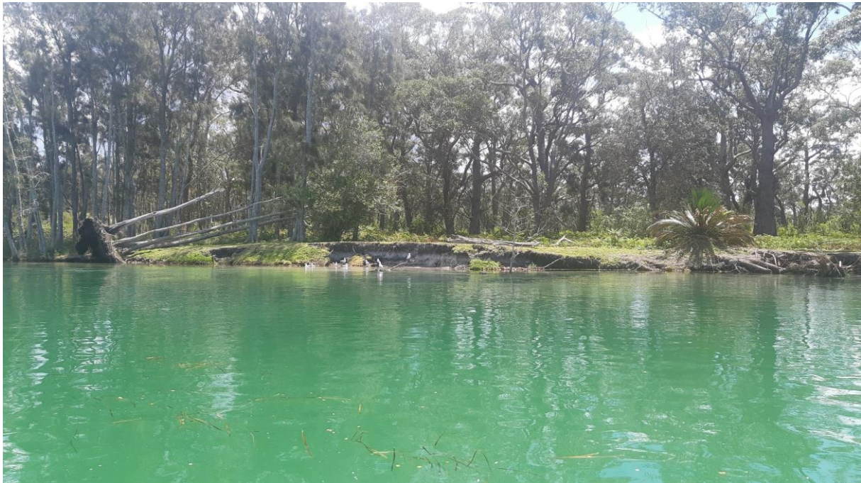
Figure 4-34 – Area upstream of Christian’s Minde. Note undermining of large trees and formation of vertical erosion scarp (7 December 2021). Site reference S006.
