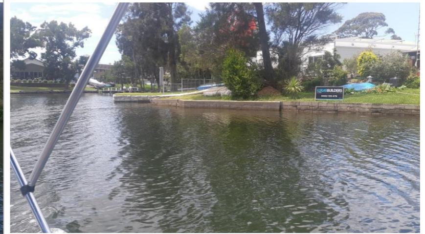
Damaged seawall at The Quays Site Ref S010
