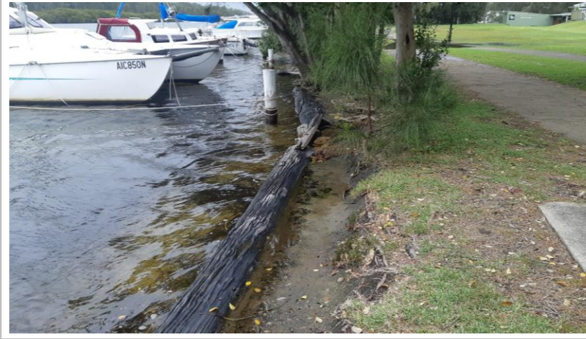
Timber log foreshore protection with erosion behind, near Sussex Inlet RSL
