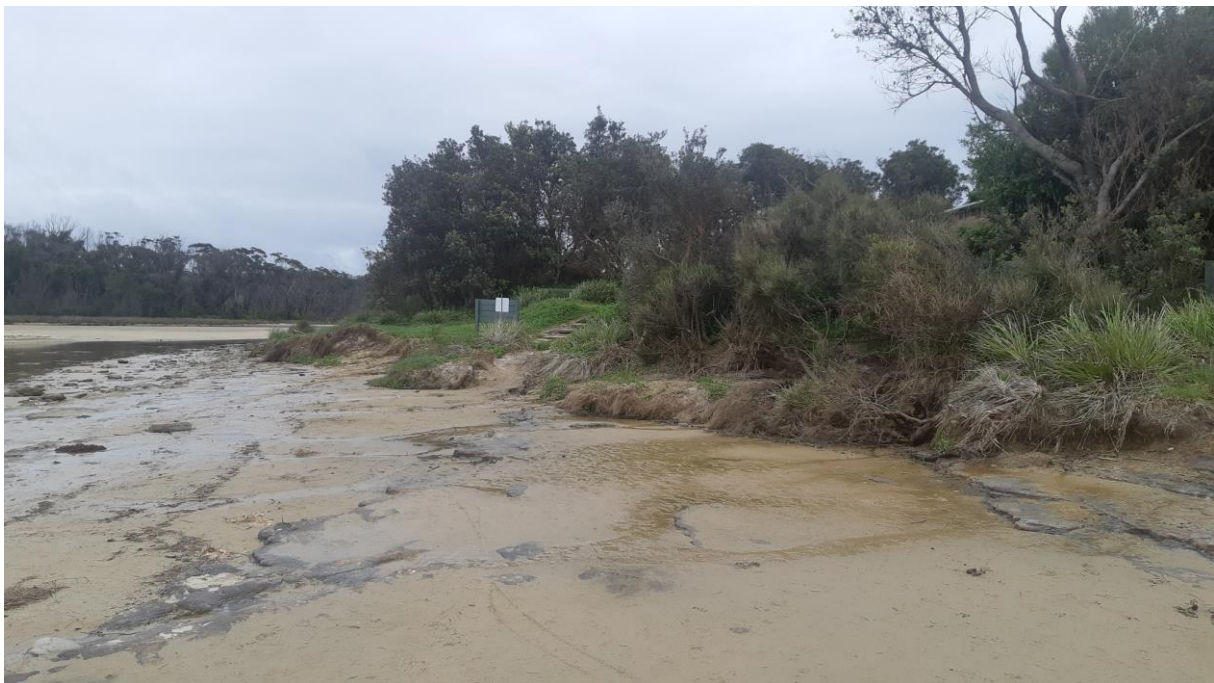
Figure 6-3 – Active erosion at beach access from carpark (1 December 2021). Site reference BC01.
