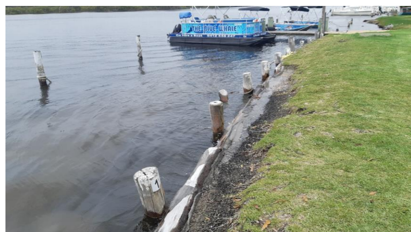
Sinkholes behind timber seawall, treated by filling with gravel Site Ref S004
