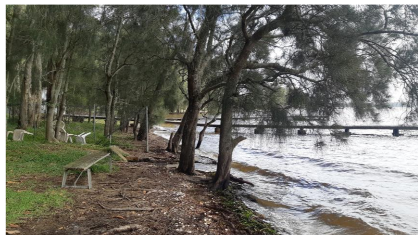
Erosion near stormwater outlet at Blackett Reserve. [REDACTED] Site Ref STB01
