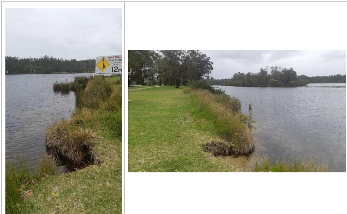
Figure 4-24 – Erosion at Sussex Inlet, just north of Sussex Marine Centre (27 November 2021). Site reference S005.
