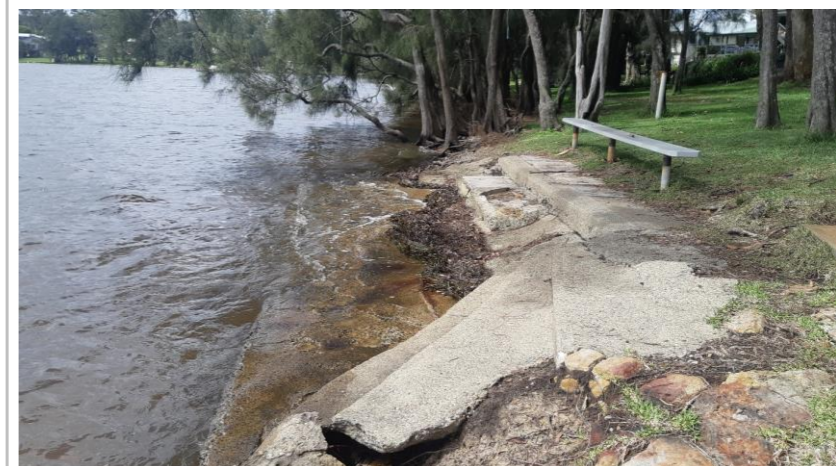
Concrete-lined foreshore with seating at Blackett Reserve. Note undermining of slab by erosion Site Ref STB01
