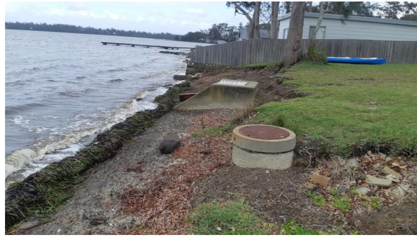
Foreshore erosion threatening sewer infrastructure at Wharf Road, Erowal Bay Site Ref EB01
