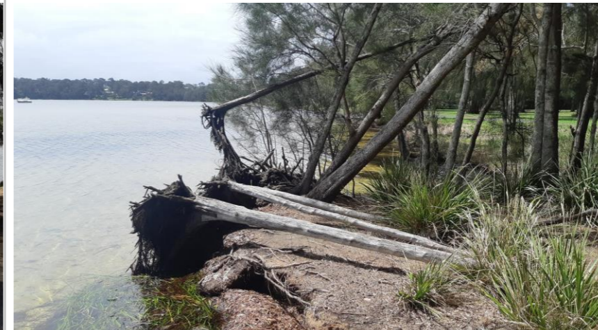
Erosion due to undermining of trees at Paradise Beach Site Ref PB02
