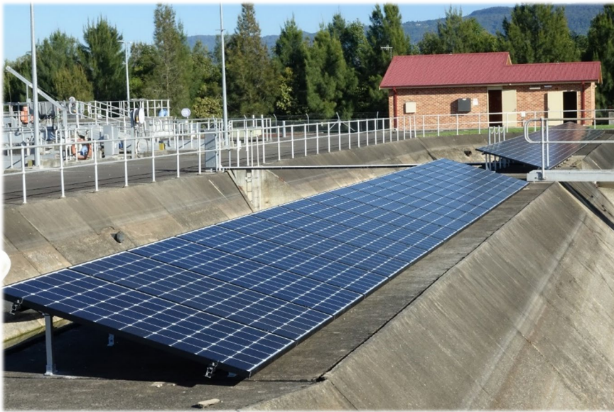
Solar photovoltaic (PV) panels installed on a disused part of the Berry Wastewater Treatment Plant helping to lower grid electricity costs and generate renewable energy to operate the plant.
