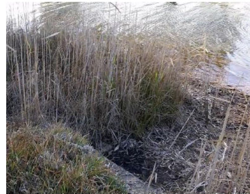
d) Blockage of stormwater outlets by sediment from catchment runoff, Riviera Keys Island Reserve, Sussex Inlet (photo courtesy Riviera Keys Island and Reserve Parkcare)
