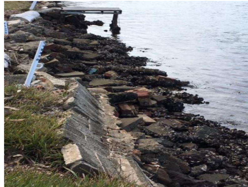
b) Foreshore erosion, Alamein, Sussex Inlet
