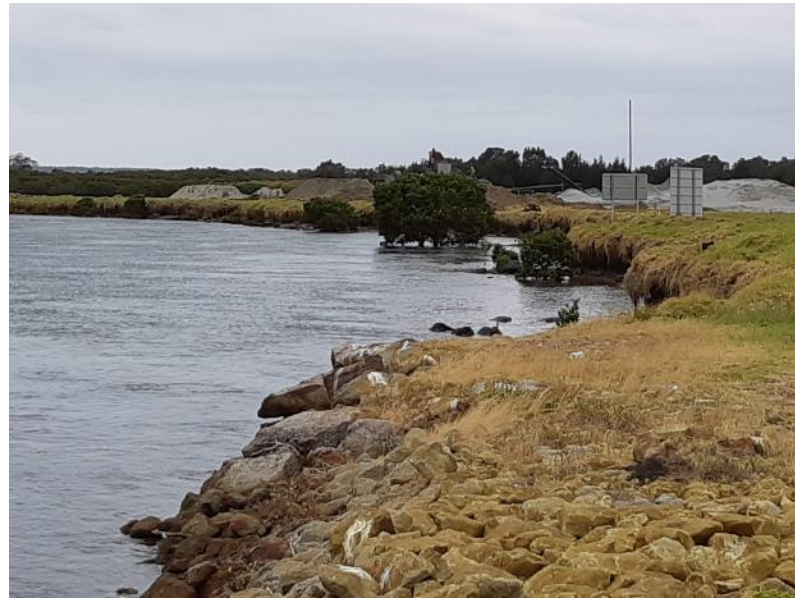
a) Bank erosion at Berrys Canal due to ongoing channel adjustment
