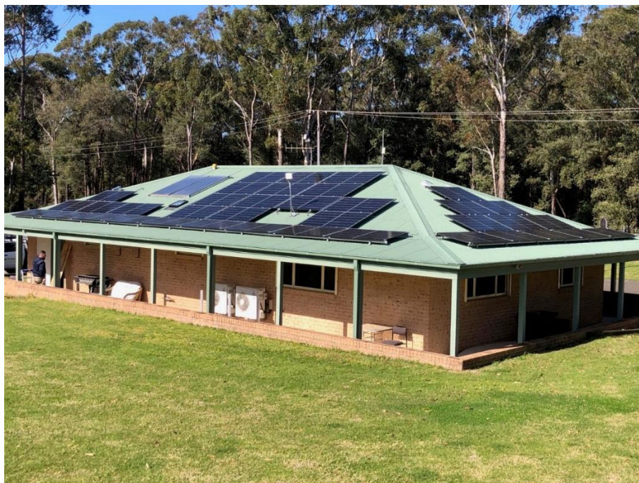
A 20-kW solar PV installation at St Georges Basin Wastewater Treatment Plant
