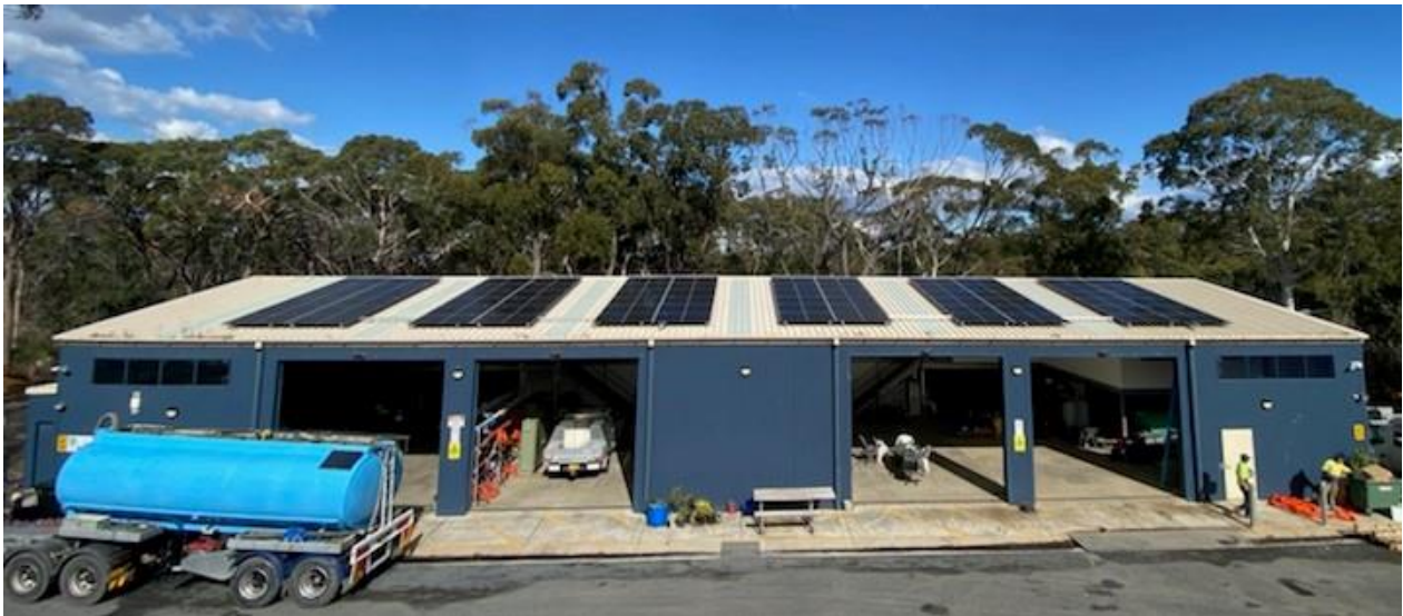
A 30-kW solar PV system installed on the Shoalwater Shed roof at the Ulladulla Works Depot in 2022
