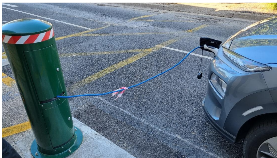
Charging a Council-owned EV at the Ulladulla Works Depot
