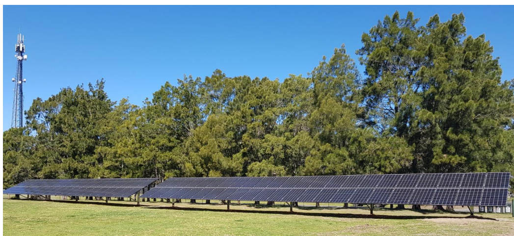
Above - A 31 kW solar PV system installed by Council at the Sussex Inlet Wastewater Treatment Plant.
