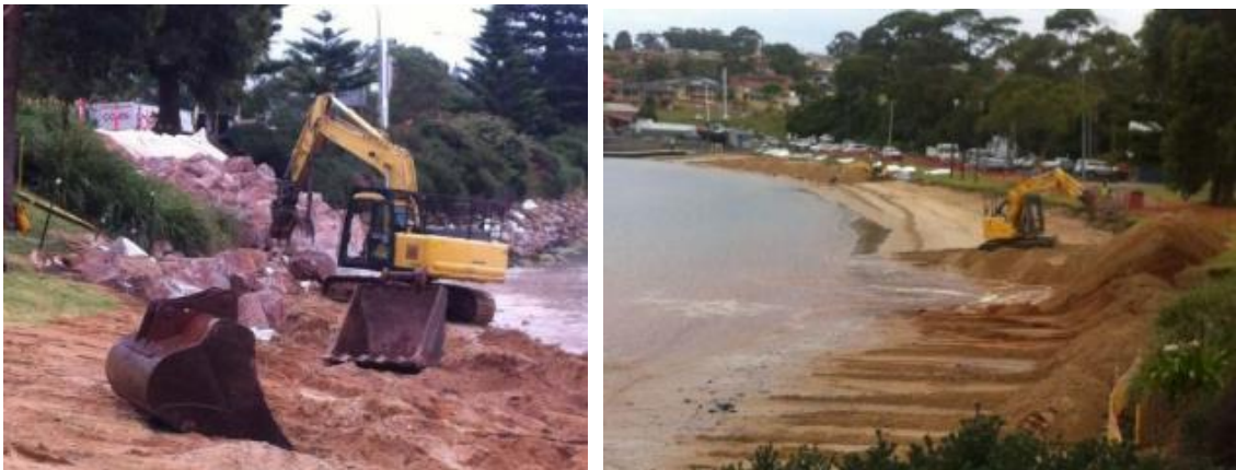
Figure 2-5 Revetment repair works (left) and beach scraping (right), after the June 2016 ECL. Image source: SCC.
