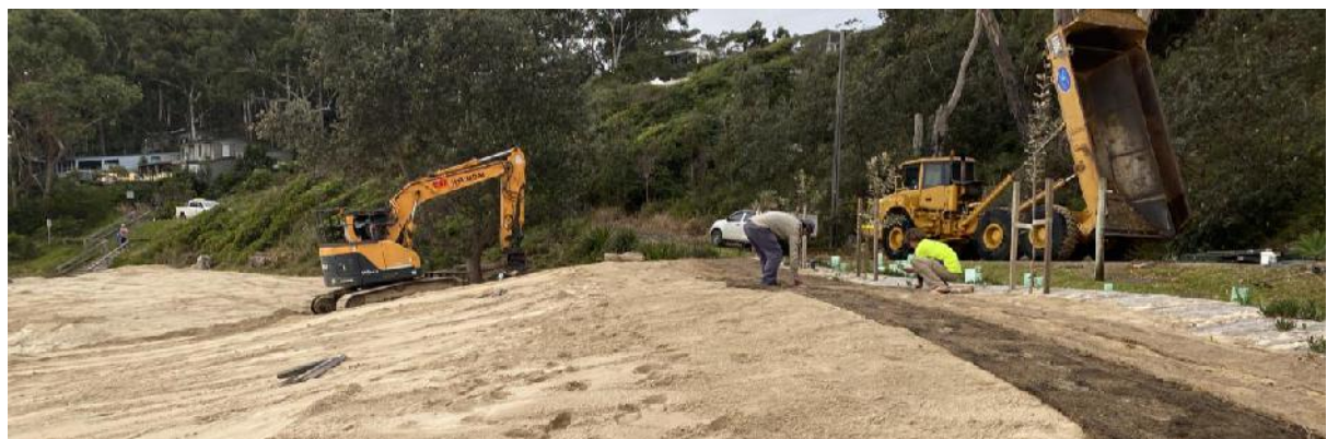
Figure 2-9 Beach scraping and dune rebuilding works undertaken by Council at Narrawallee Beach in June 2022. Image source: SCC
