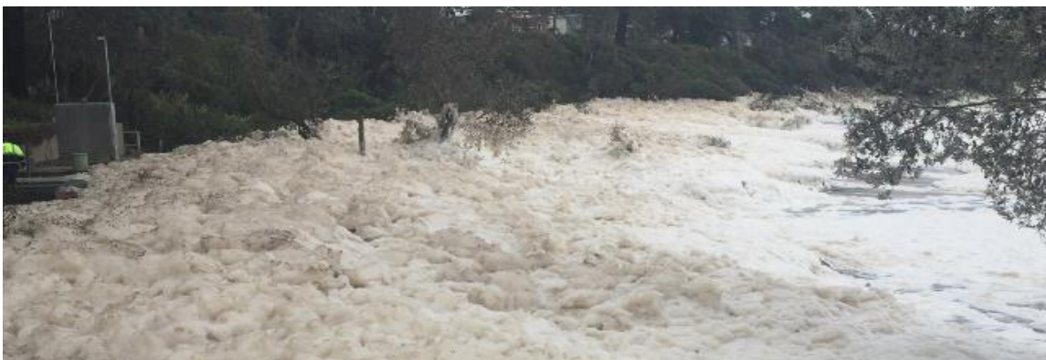
Figure 2-6 Wave run-up and coastal inundation of a sewage pump station at Narrawallee Beach during the June 2016 ECL. Image source: SCC.
