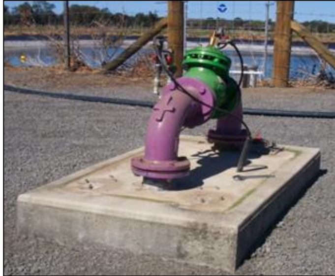
Figure 2-4 – Photograph of Farm flow control valve
