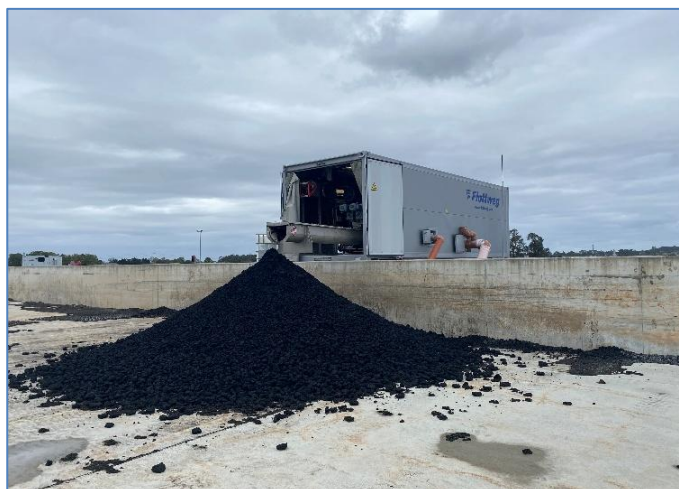
Figure 2-8 – Photograph of Council's Permanent centrifuge at Nowra WwTP
