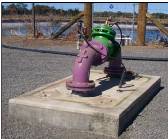
Figure 2-4 – Photograph of Farm flow control valve
