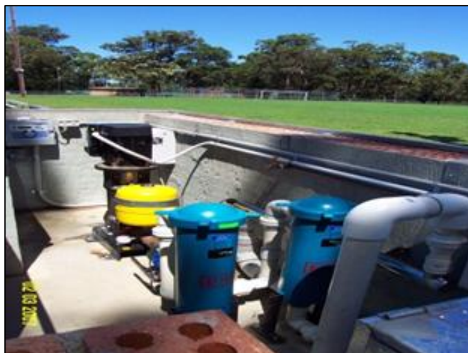
Figure 2-3 – Photograph of Pumping & Disinfection System - Huskisson Sports Field
