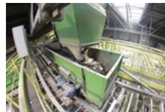
Autoclave being loaded
