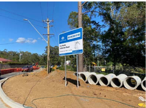
Completed kerbing on the new roundabout at Illaroo Road and West Cambewarra Road as part of the Far North Collector Road. (Dec 2020, source: Shoalhaven City Council)
