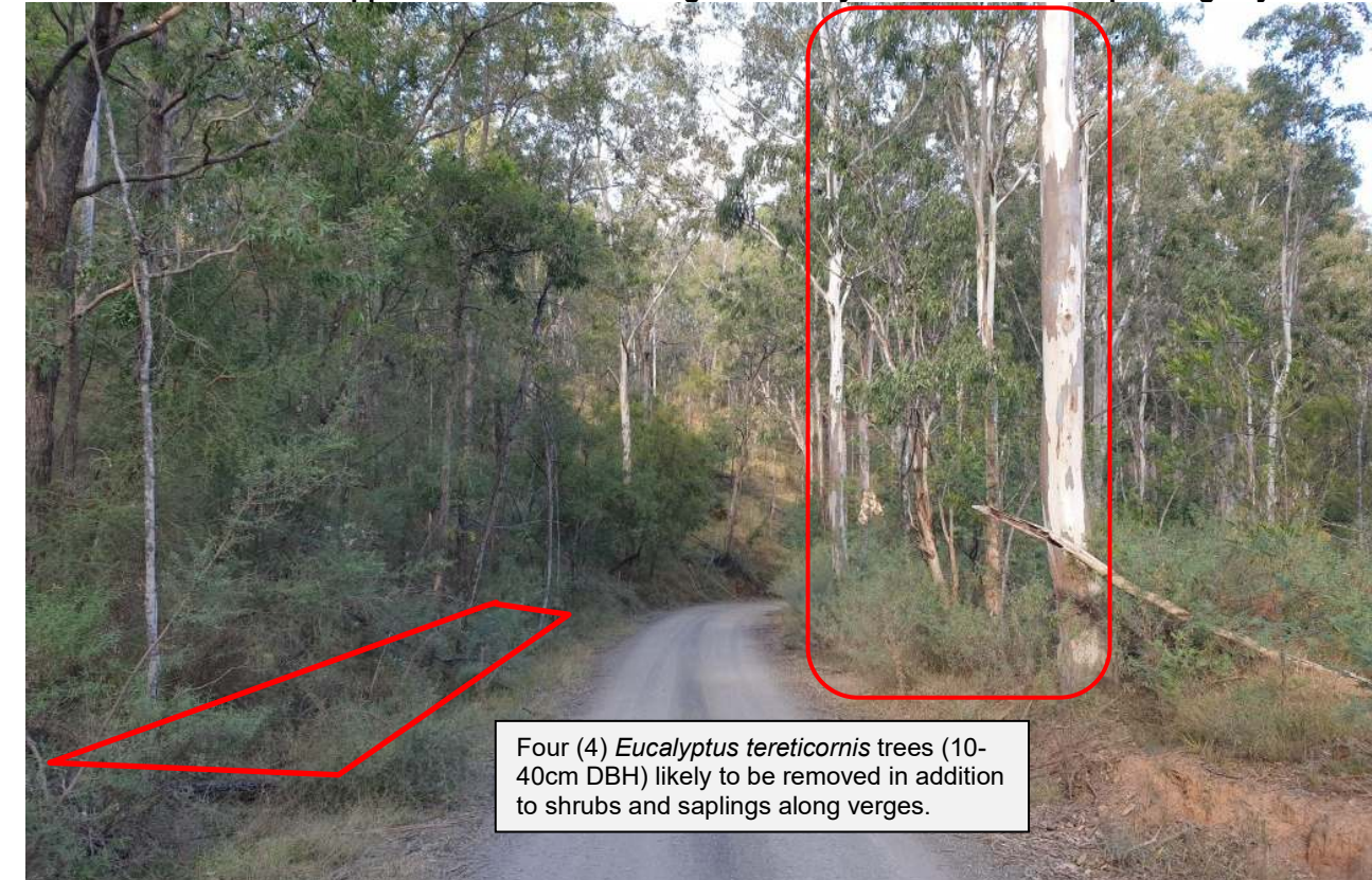
Photo 4. Access road at approx. Ch. 250 m showing trees likely to be removed for passing bay
