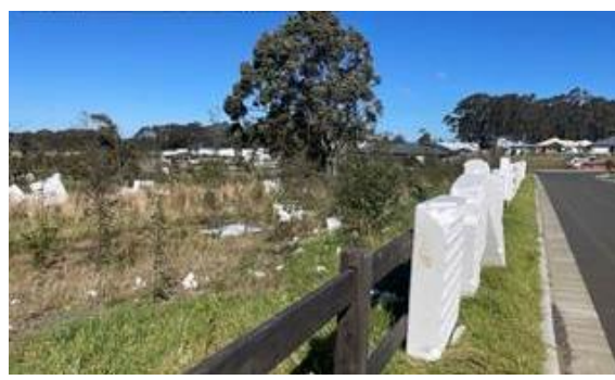
Badagarang – Pollution incident Waffle pods blown from a building site
